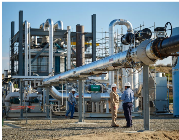
Chevron Demo Plant – flue gas line
