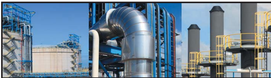
Dragon LNG commissioned its import terminal in South Wales in August 2009. With a capacity to unload 217,000 cubic metre capacity carriers and send out to the NTS 1,200,000 standard cubic metres per hour, it is one of the UK key gas supply facilities. More photos on page 2. Photos courtesy of Dragon LNG
