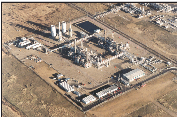
Views of the Teesside px plant, the Operating Asset to be visited in May. Photos courtesy of px(TGPP)
