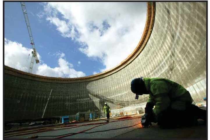
190,000m 3 LNG tank, big enough to hold the Albert Hall!
