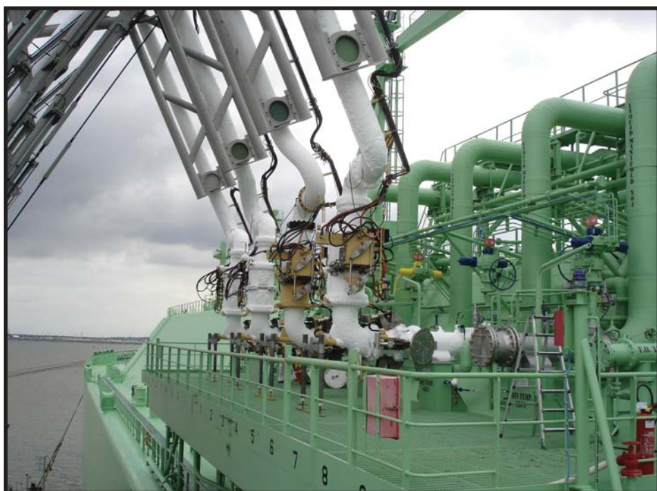
LNG Unloading Arms. For the report of the site visit to Isle of Grain see page 13. Photo courtesy of National Grid
